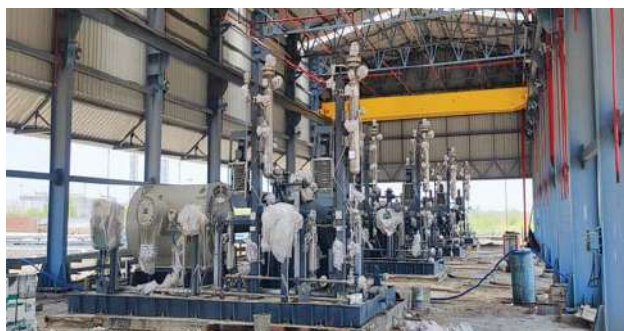
Viramgam Pump Station (MLPU Shed)
