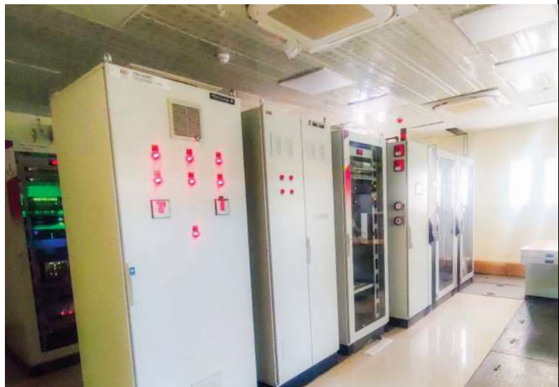
Equipment Room IOCL Bhopal
