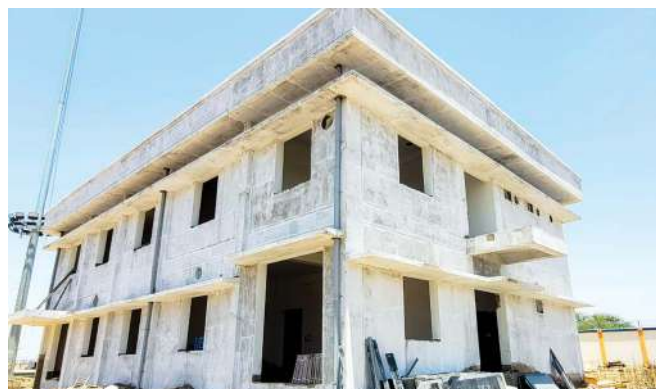
Dhar Pump Station (VFD Building)
