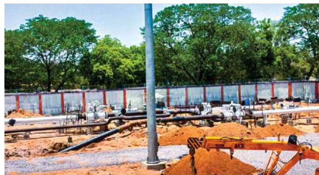
Intermediate Pigging Station (Lalitpur)
