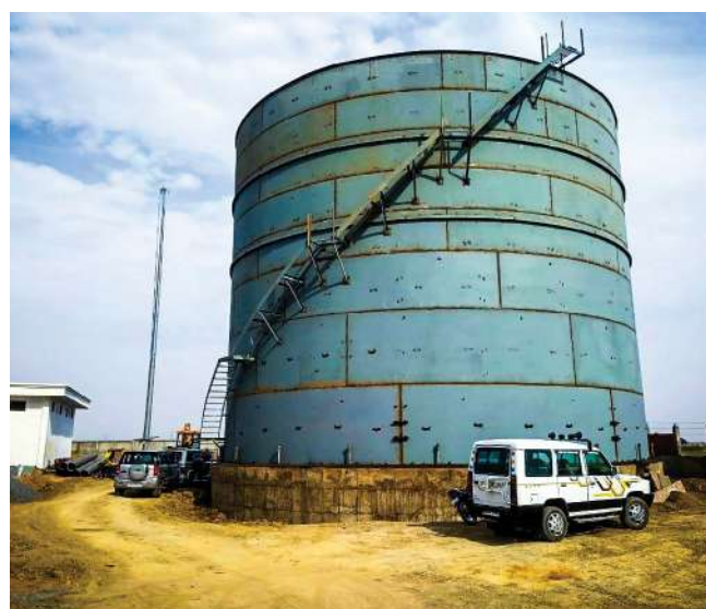
Water Tank at Intermediate Pigging Station (Jalaun)
