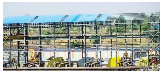
Dhar Pump Station (MLPU Shed)
